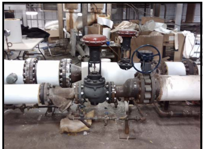
Steam Station in the Utility Plant
