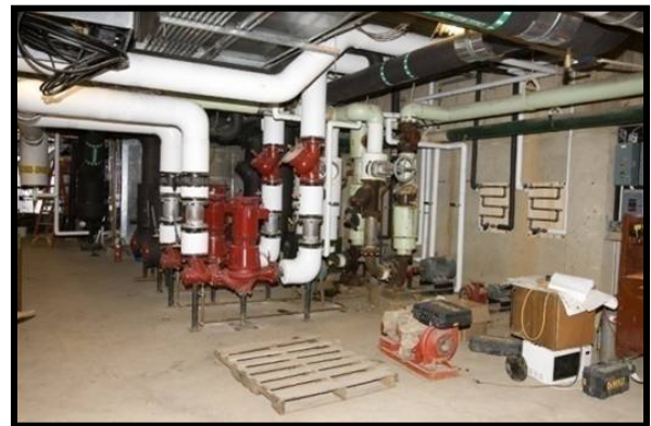
Smith Hall HVAC Mechanical Room
